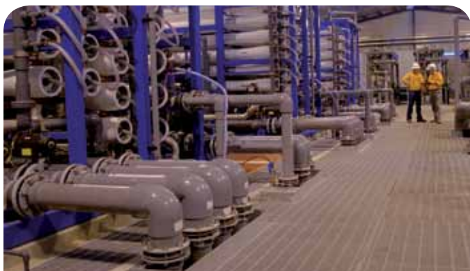
CSG water is purified at our water treatment facilities
